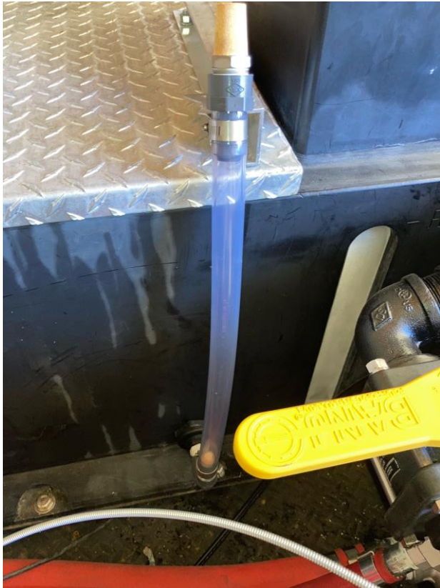
Water level site gauge, original window is no longer translucent
