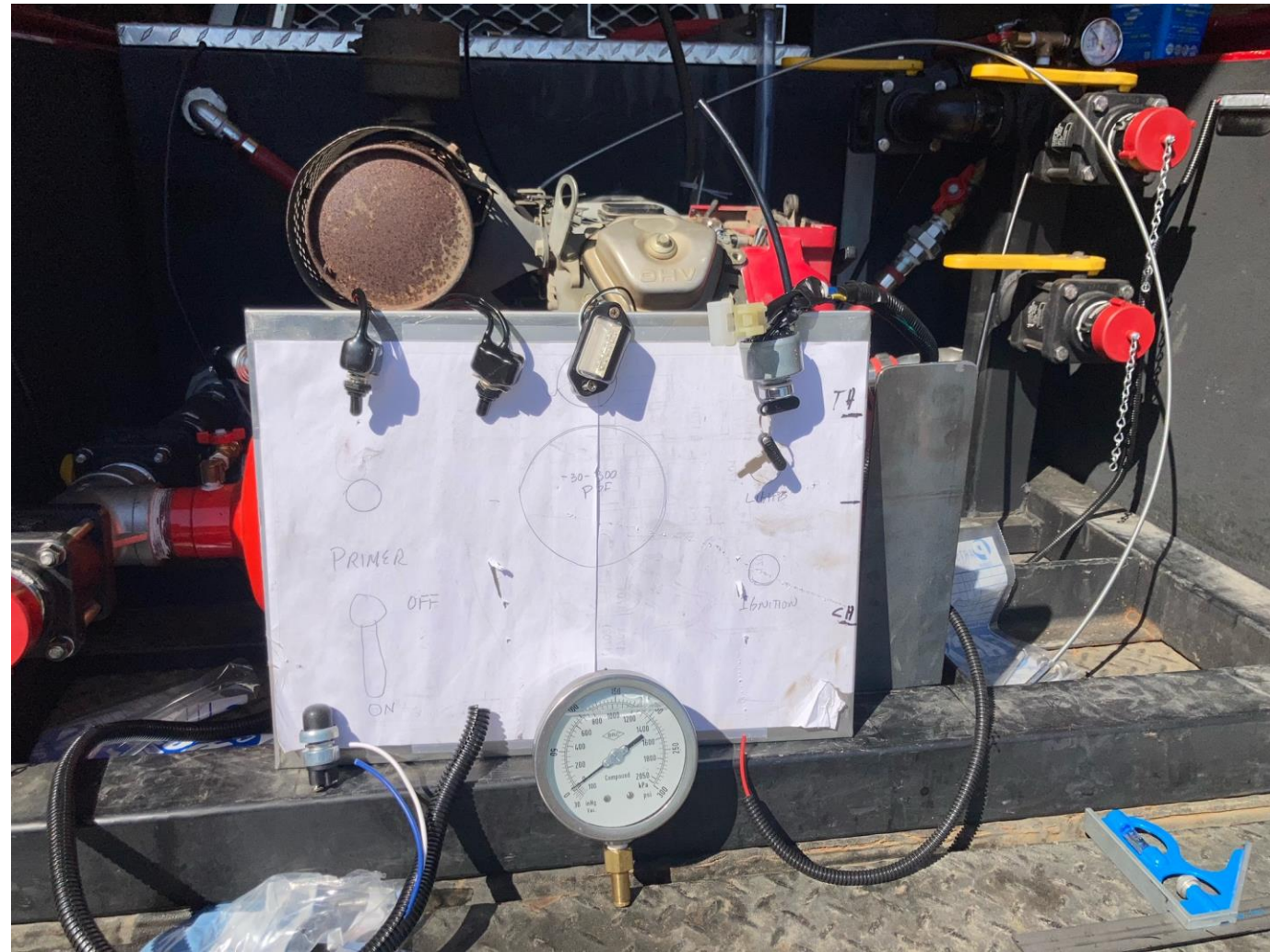
Pump panel in progress. Shows, relocated key start, switches, lights, wires, hoses, and gauges to be mounted
